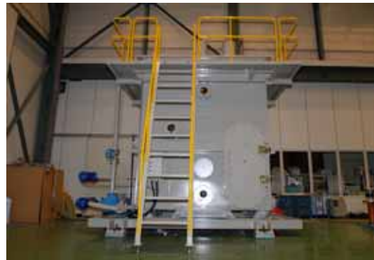
Fig. 2. Transformer for experiment.
