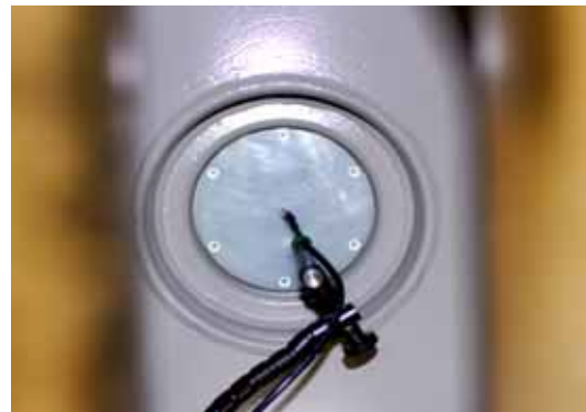
Fig. 6. Discharge source in front of sensor 8 seen between mock windings.
