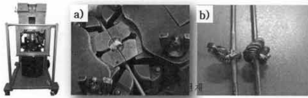
Fig. 1. The cold weld of aged Al wire. (a) welding dies and wire position, (b) cold welded Al wire before burr removal.
