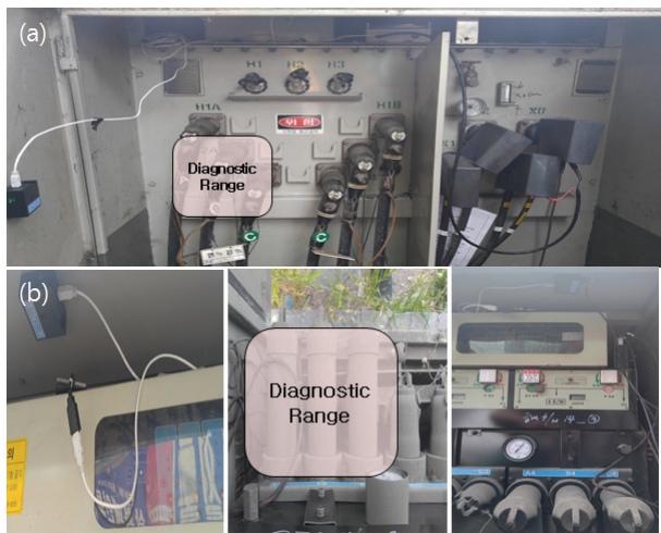
Fig. 10. Photograph of field installation.
