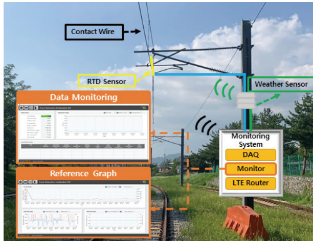
Fig. 3. Picture of monitoring system for catenary frost or freezing.
