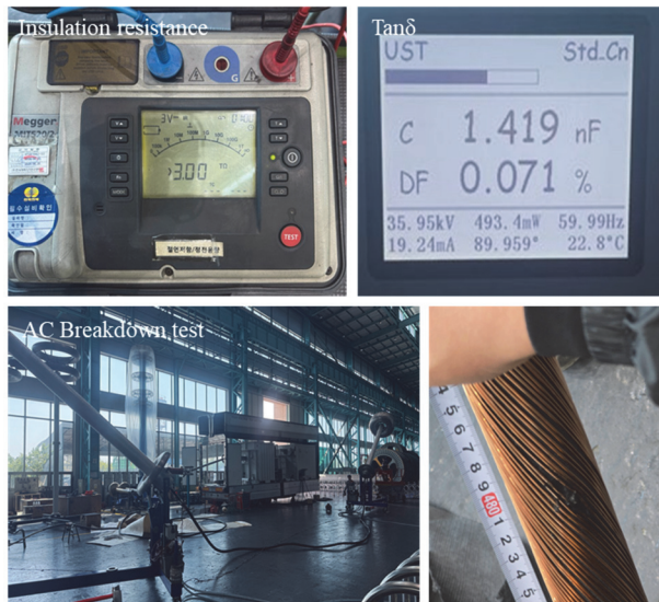
Fig. 8. Photographs of the cable insulation performance evaluation.
